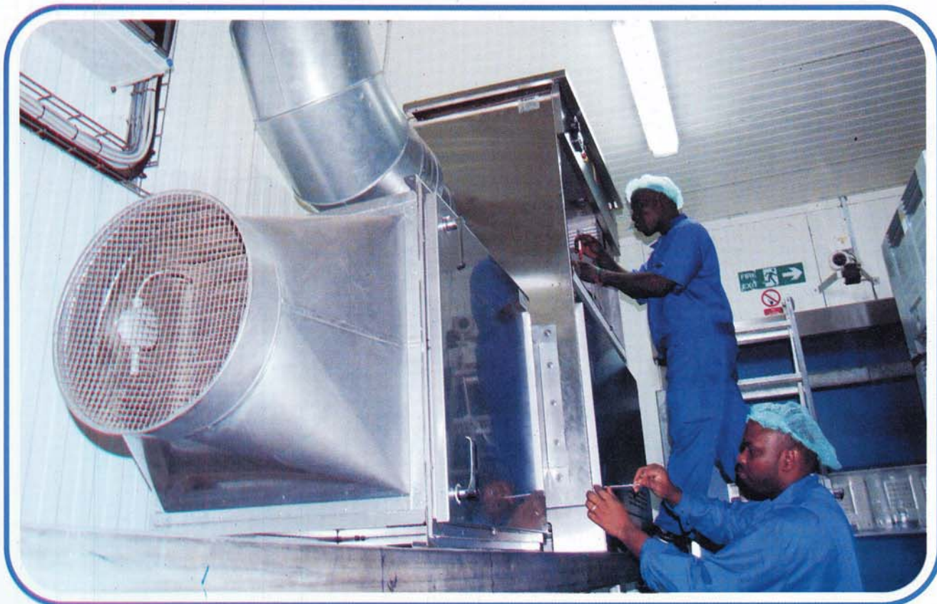
New dehumidifier equipment.
