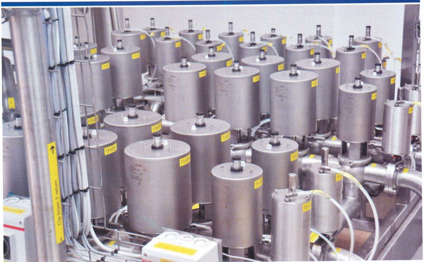
Automatic valve station.
