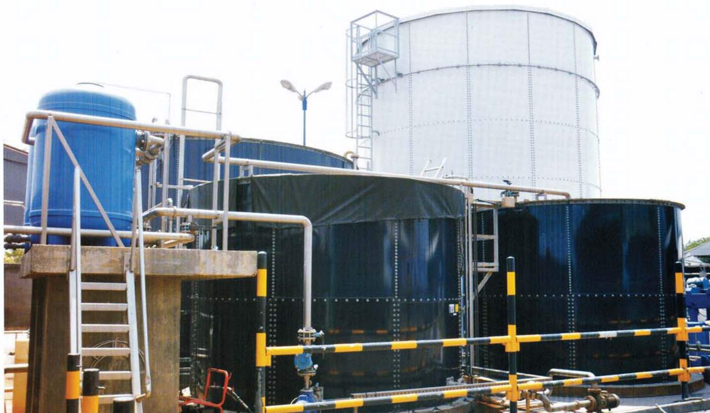
Waste water treatment plant.
